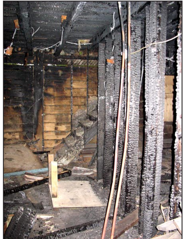
Interior fire damage, Barber House
