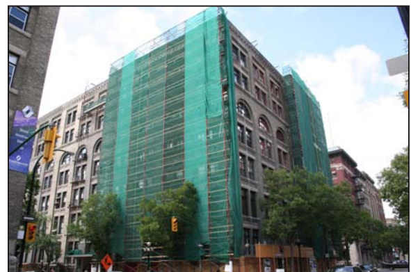
Scaffolding used during exterior cleaning and repairs on the Merchant's Building, 250 McDermot Avenue, July 2008
