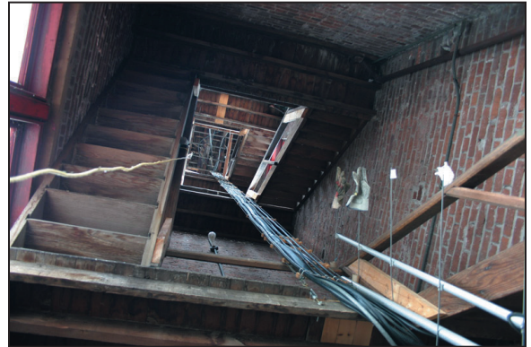
St. Vital Fire Hall and Police Station, hose drying tower with wooden staircase
