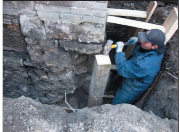
Worker hammering in a 6x6 post for temporary support of the southeast corner during foundation repairs at 88 Adelaide Street
