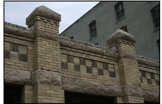
Detail of north façade of the Toronto Hide and Wool Company Building
