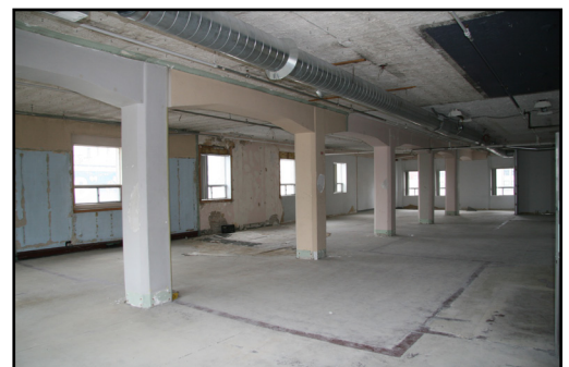
Concrete supports on the 3rd floor of the Keewayden Block (Jacob-Crowley Building)
