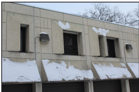
St. Boniface Police Station/Jail/County Courthouse, 227 Boulevard Provencher, fenestration on the east side, 2020. (M. Peterson)
