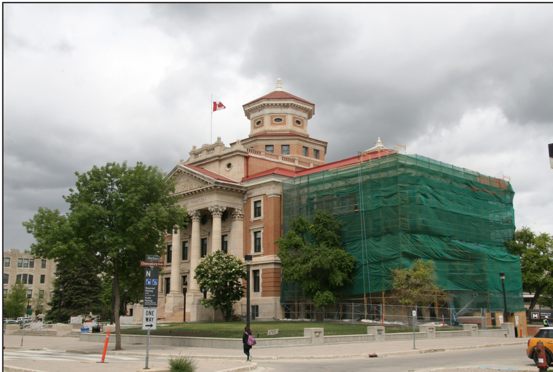
Administration Building, University of Manitoba, 66 Chancellors Circle, south and east façades, 2021. (G. Menzies)
