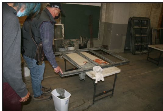
90 Annabella Street, J.R. Watkins Company Factory and Warehouse, window repairs, 2021. (G. Menzies)
