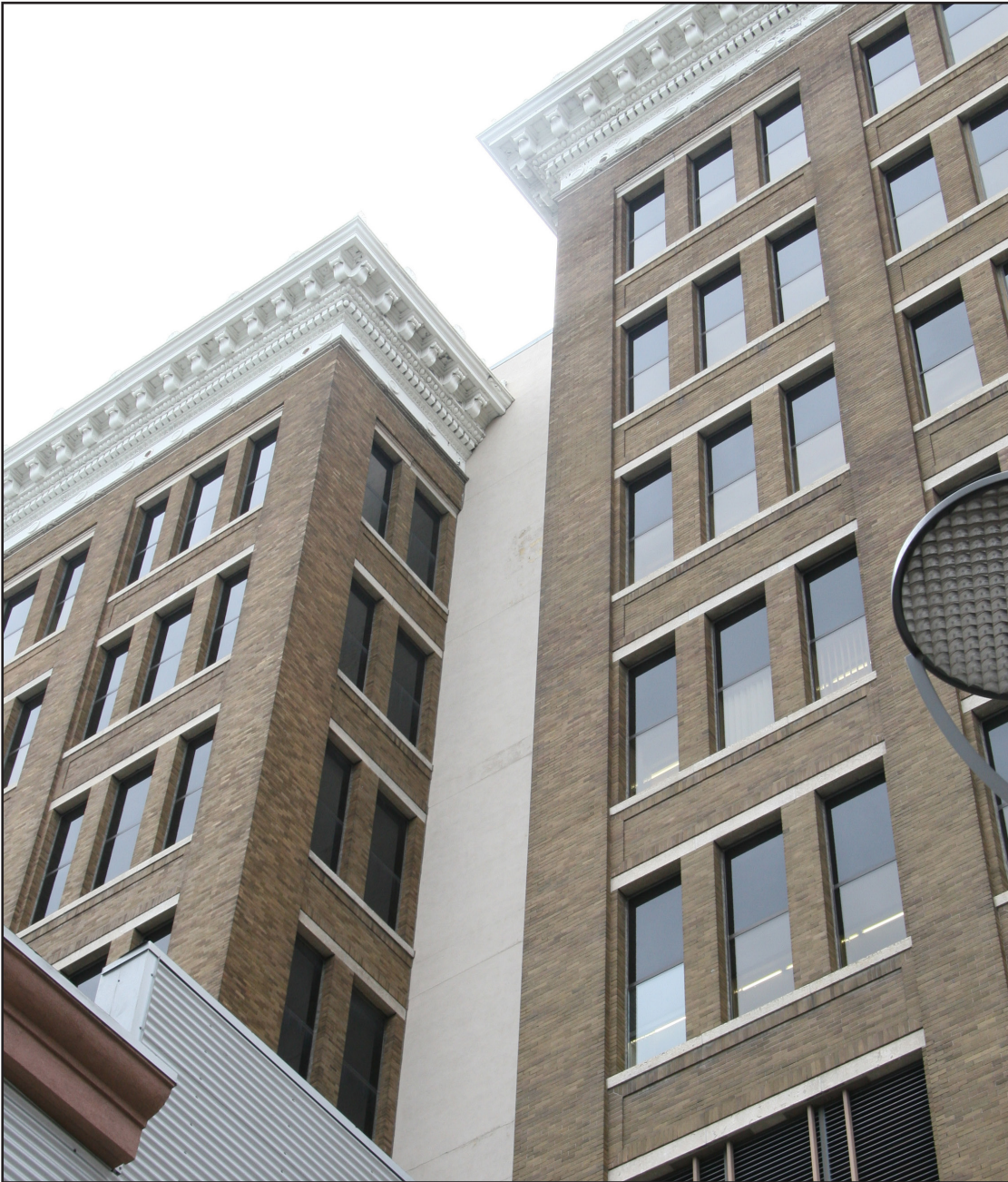
Detail of the north façade, T. Eaton Company Mail Order and Catalogue Building, 333 St. Mary Avenue, 2016. (M. Peterson)
