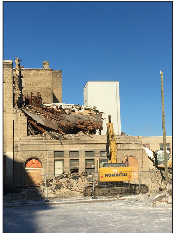
Thomas Scott Memorial Orange Lodge, 216 Princess Street, southeast corner, February 2020 demolition in progress. (M. Peterson)
