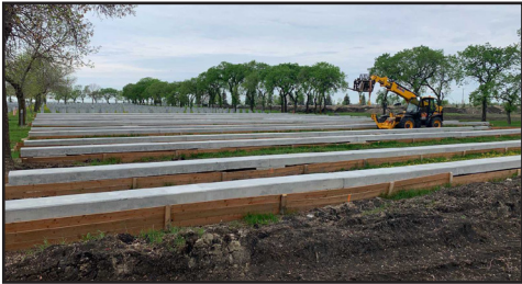
New concrete beams in the Field of Honour, Brookside Cemetery, ca.2010. (Reproduced from Haywood Concrete Products Ltd. website, https://haywoodconcrete.com/project-gallery .)
