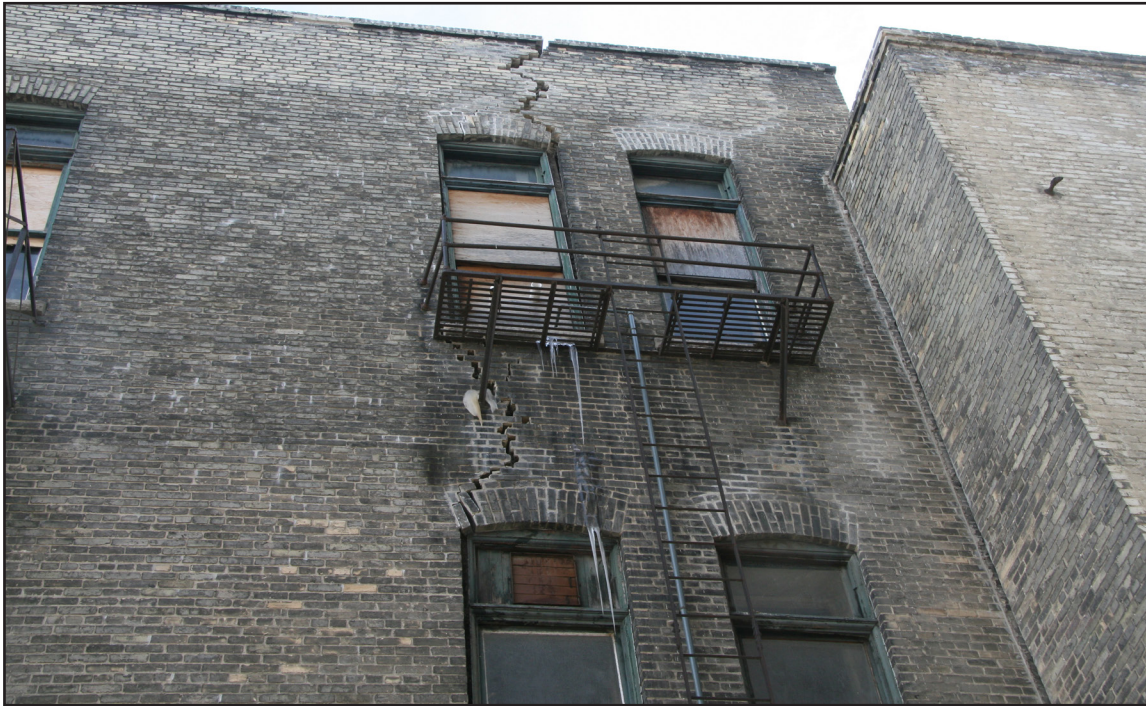
Thomas Scott Memorial Orange Lodge, 216 Princess Street, rear (west) façade showing significant brick cracking, 2020. (M. Peterson)
