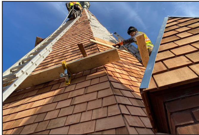
Workers installing wood shingles on the tower at Calvary Temple, 400 Hargrave Street, 2021. (G. Menzies)
