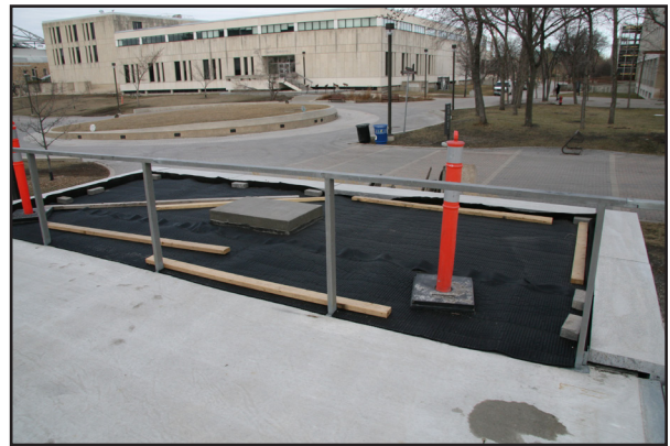
J.A. Russell Building, University of Manitoba, 83 Dafoe Road, rusting handrail prior to restoration, 2020. (G. Menzies)
