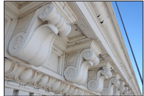
Detail of the metal cornice, T. Eaton Company Mail Order and Catalogue Building, 333 St. Mary Avenue, ca.1999. (City of Winnipeg)
