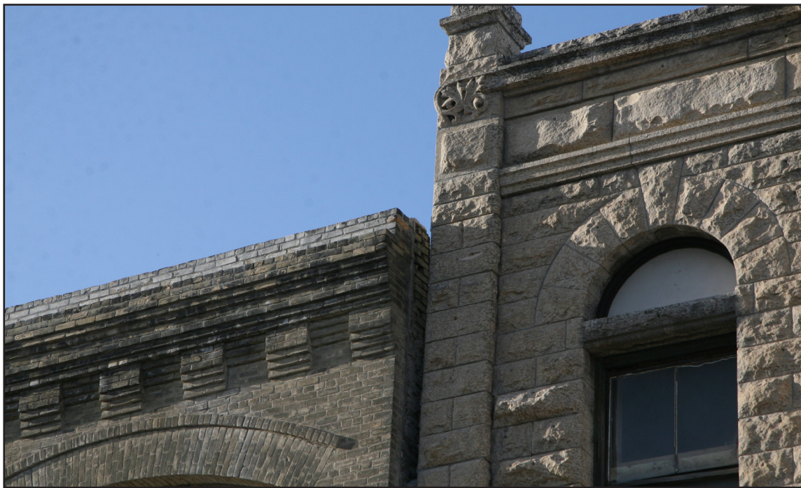
Thomas Scott Memorial Orange Lodge, 216 Princess Street, southeast corner, showing the building pulling away from the neighbouring structure, 2020. (M. Peterson)
