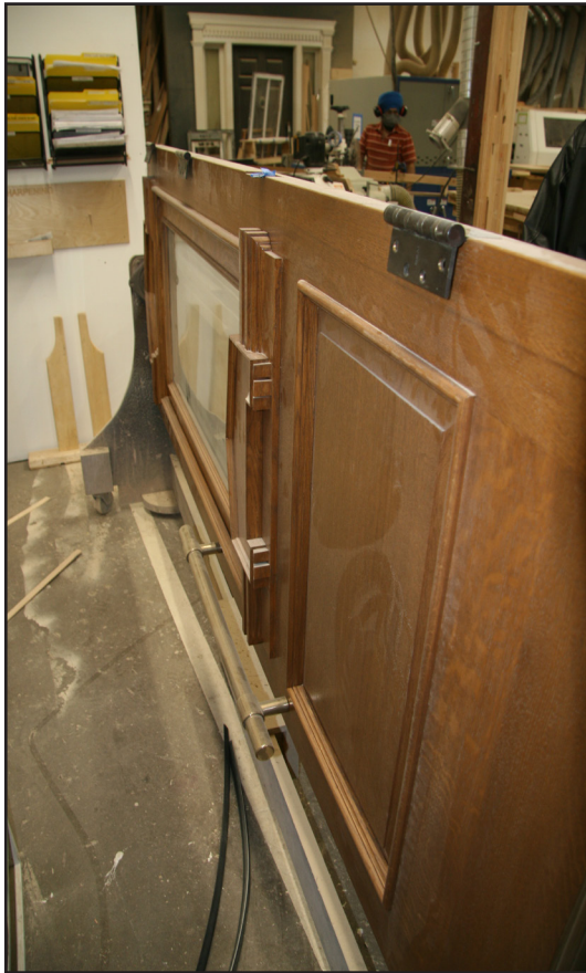
Université de Saint-Boniface, St. Boniface College, 200 Avenue de la Cathedrale. Door at the Yarrow Sash and Door shop, 2021. (City of Winnipeg)
