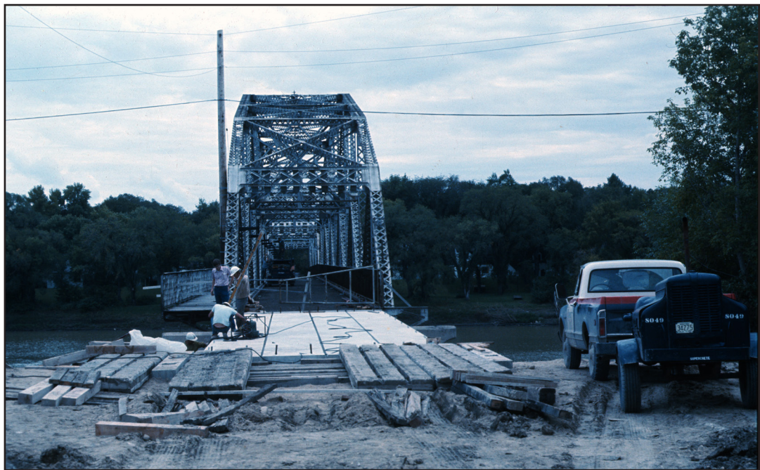
The Elm Park Bridge, 1975, as City workers complete repairs to the deck to allow for pedestrian traffic. (Historical Buildings and Resources Collection)
