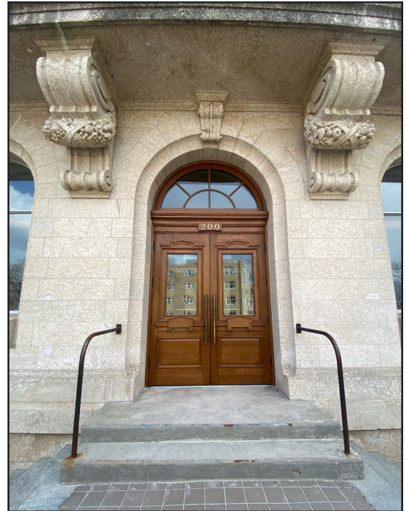
Université de Saint-Boniface, St. Boniface College, 200 Avenue de la Cathedrale, new door installed, 2021. (City of Winnipeg)
