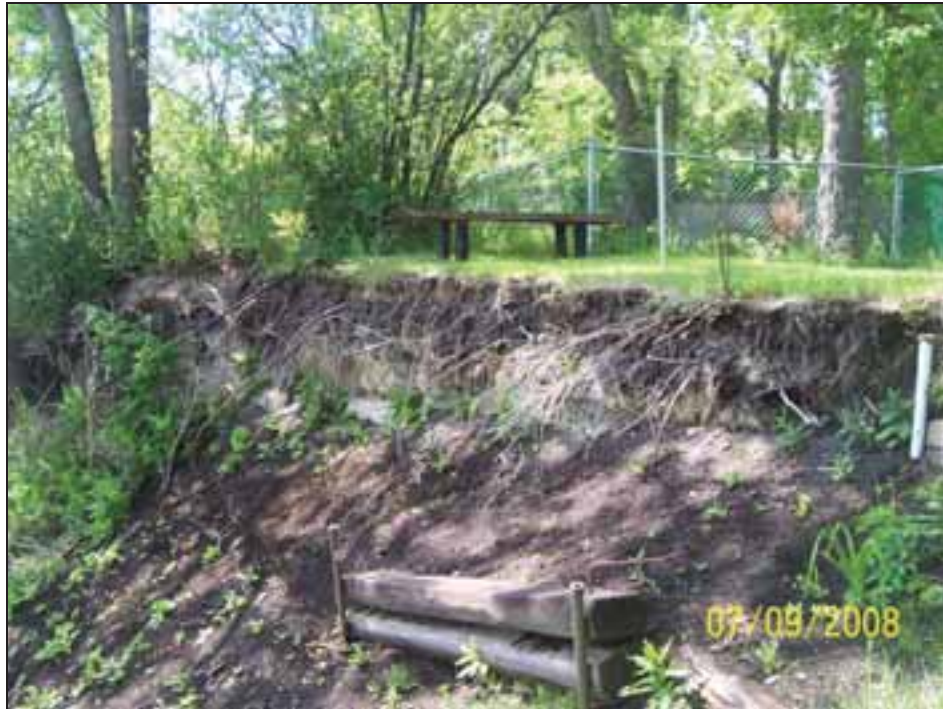
Photo 5 – Riverbank instability at property located immediately upstream of Elm Park Foot Bridge (BDI Location).
