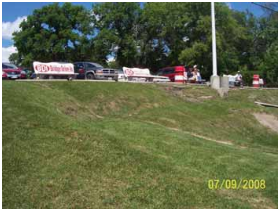
Photo 6 – Top of bank area of proposed BDI outfall location. Note: Evidence of historic bank movement near top of bank.
